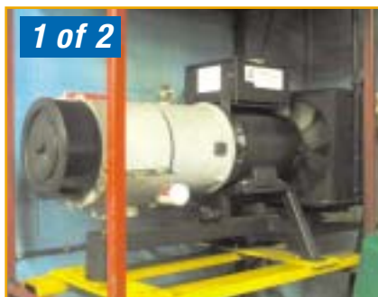
COMPAIR 40 HP AIR COMPRESSOR
